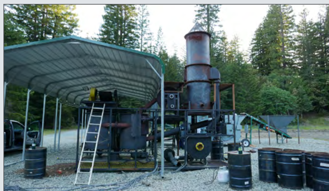
Figure ES-9. This relocatable gasification system was set up for Redwood Forest Foundation, Inc. in Andersonia, California in 2017 and is an example of a moderate-scale system. (Photo: Arne Jacobson)
